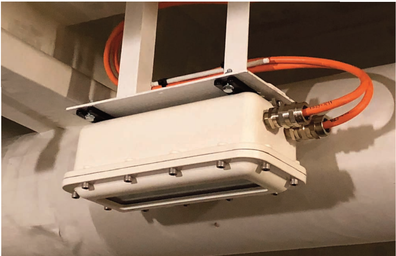
Italian Navy c6259 LSS Vulcano -PEX explosion proof led fixtures installed on board
